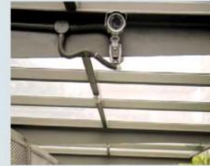
One of the 35 CCTV units around the canopy walk.
